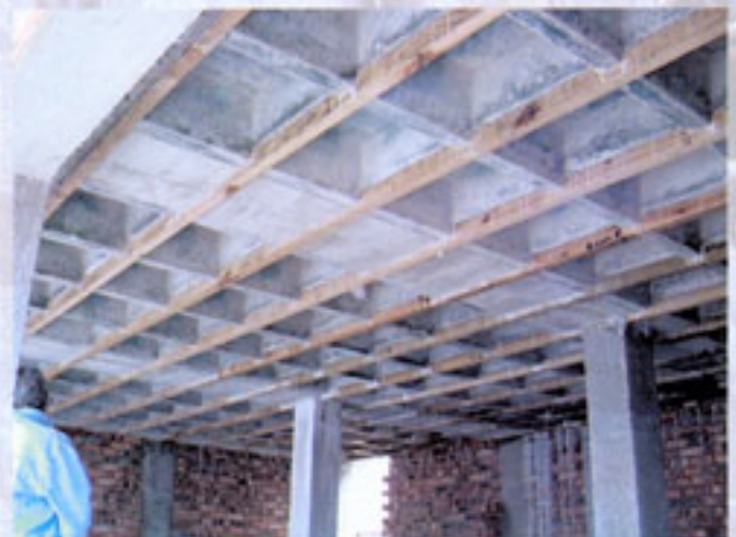
Holes can be drilled through the wooden purlins for the electric conduit and plumbing pipes.
