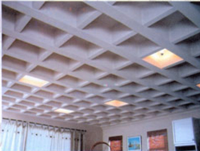
The ceiling of a house in Ysterfontein painted and fitted with lights.
