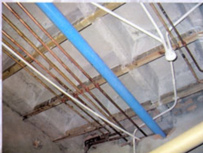
Plumbing and electrical services fixed to the underside of the wooden purlins.
